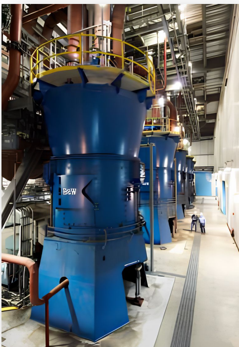
B&W Coal Grinding Machine
